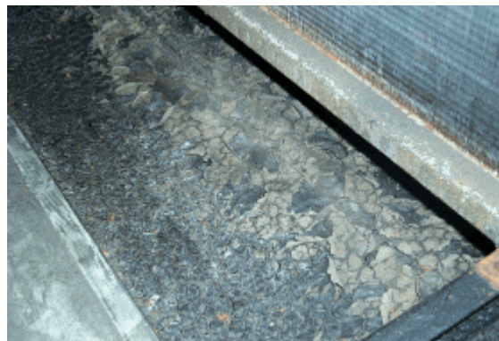
Batteries with dirt and corrosion
